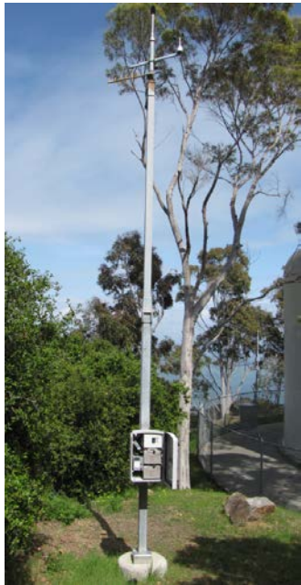
Site 7 – Permanent Monitor
